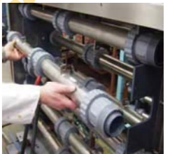
★压载水处理装置 Evoqua Water Technologies
