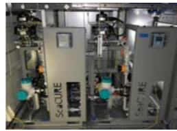
★压载水处理装置 Evoqua Water Technologies
