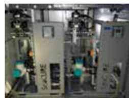
★Ballast Water Management System Evoqua Water Technologies
